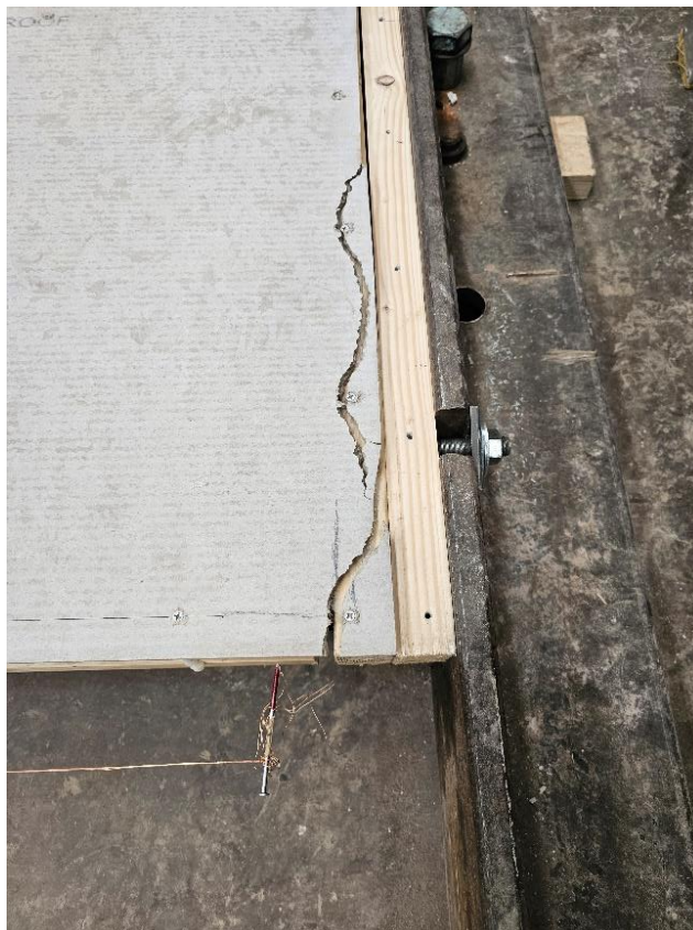
Plate 2 – Typical Mode of Failure (1)
