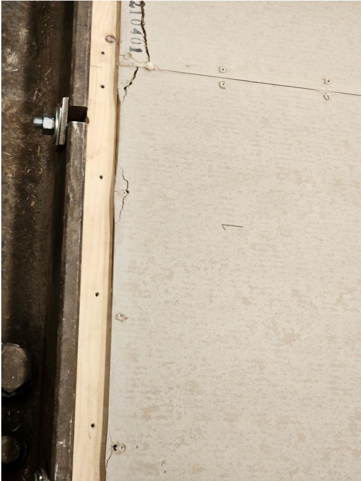
Plate 3 – Typical Mode of Failure (2)
